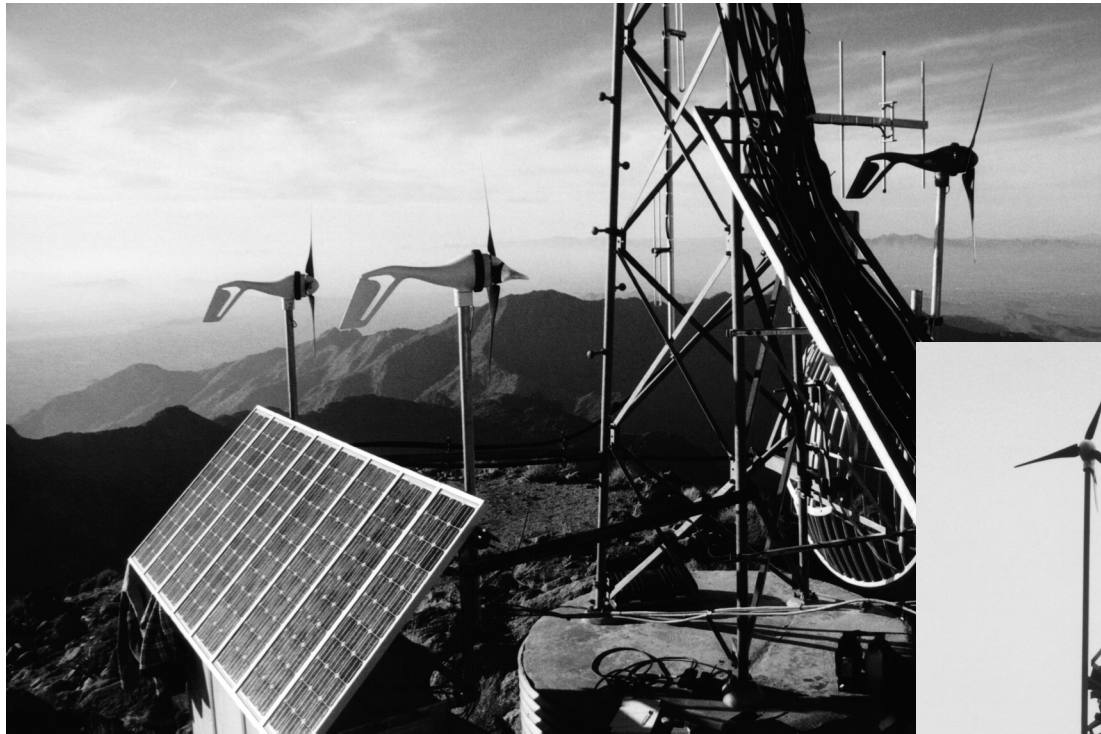
Three Air Industrial modules combined with PV provide power for a cell phone transmitter in the mountains near Phoenix, Arizona.
